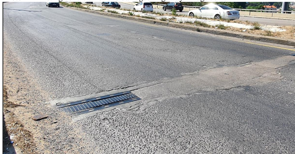
Photo 1 - Existing condition of one damaged Highway Bridge Joint
