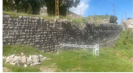
Deteriorated Stone Wall
