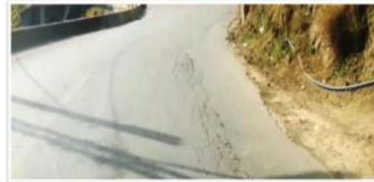
Damage in asphalt caused by fires burning
