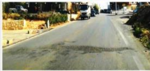
Moderate alligator cracks
