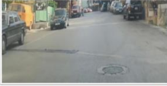
Half road width interceptor and bad manhole mortar
