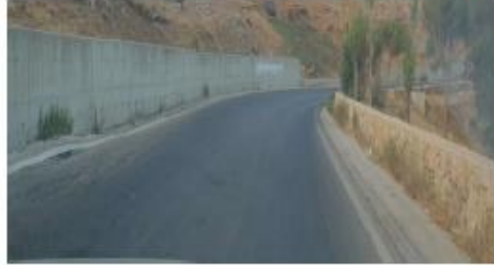
Severe deterioration in pavement structure
