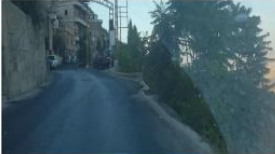
Missing safety barriers
