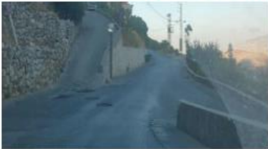
Irregular and narrow section Mismatched level manhole covers
