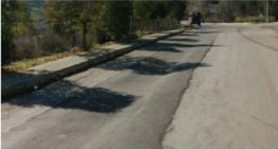
Bad trench compacting
