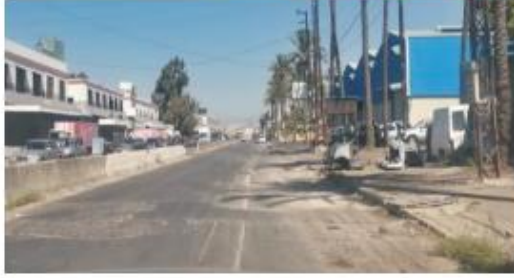
Poor Asphalt repair, and sunken utility trench
