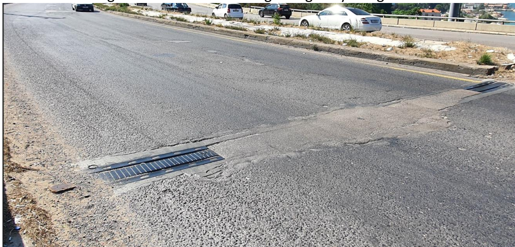
Photo 1 - Existing condition of one damaged Highway Bridge Joint
