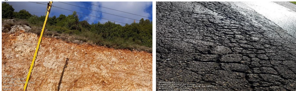
Figure 1-2 Faults, Erosion Risks and Road Cracks
