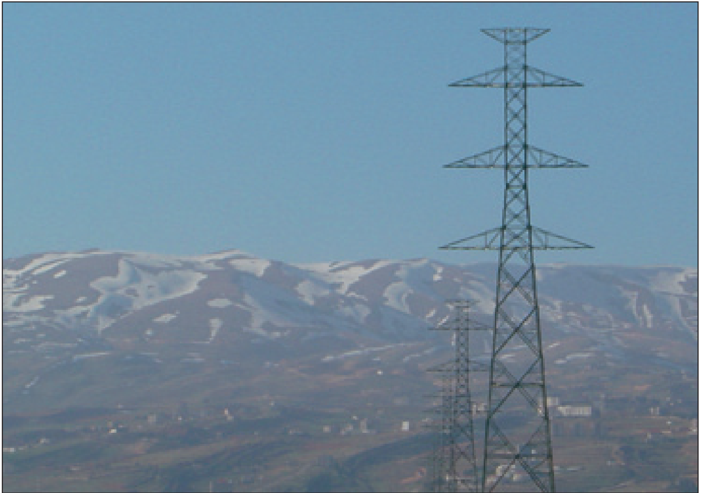
Seven countries interconnection network (400 KV)
