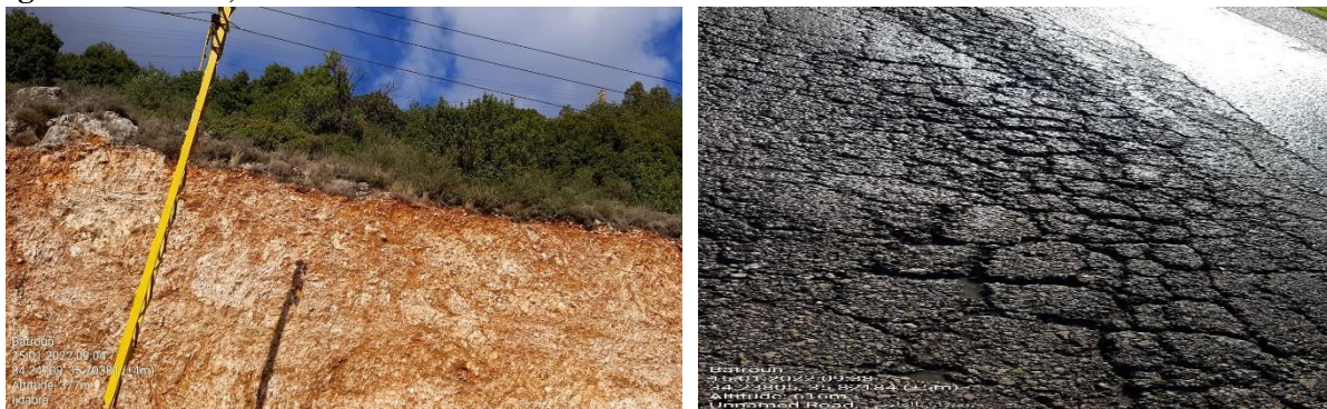
Figure 1-2 Faults, Erosion Risks and Road Cracks
