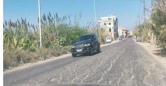
Moderate to Severe alligator cracks in the
