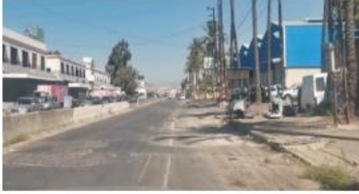
Poor Asphalt repair, and sunken utility trench
