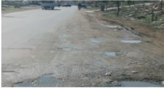
Deep pavement damage due to water infiltration
