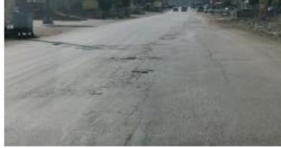
Deep pavement damage due to water infiltration
