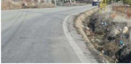
Obstructed channel presenting high risk in its shape to the road users
