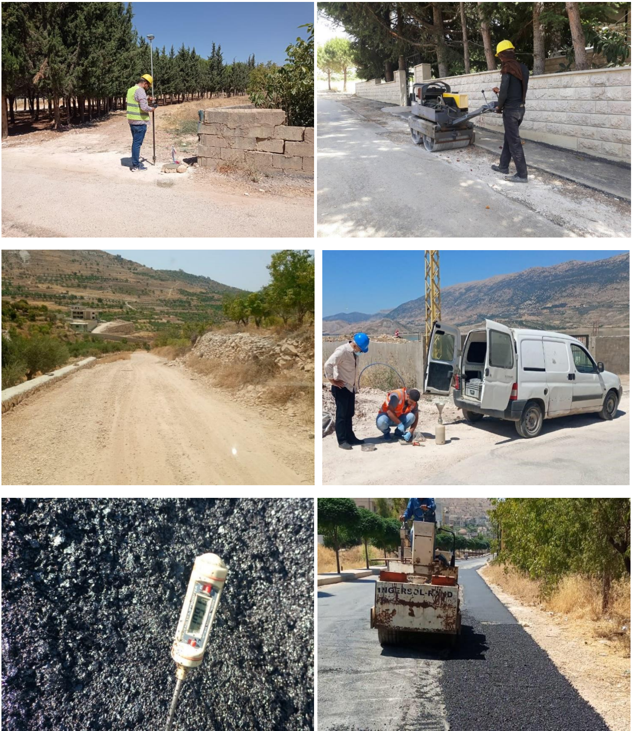
Figure 2: Site pictures from upper left to right (Surveying, Compaction of the bedding material, Preparing bedding material and surfaces before asphalt laying, Sampling for compaction test, Testing the temperature of the asphalt delivered to site, Asphalt compaction).
