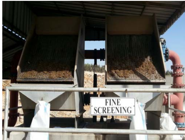
Figure 3-1 Fine Screening Unit
