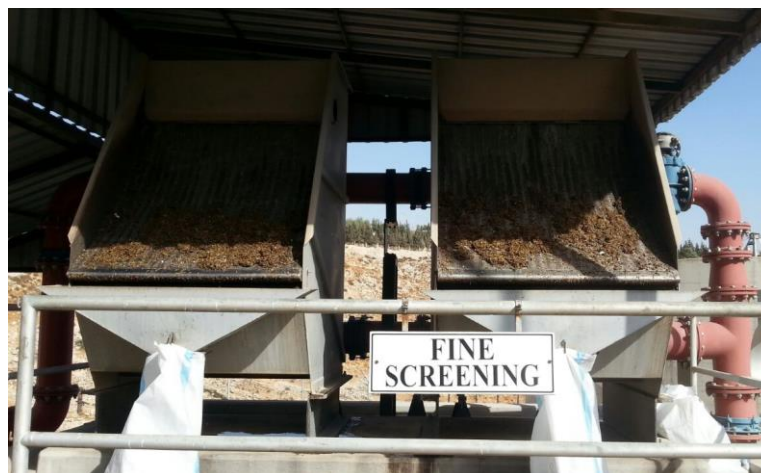
Figure 2-1 Fine Screening Unit
