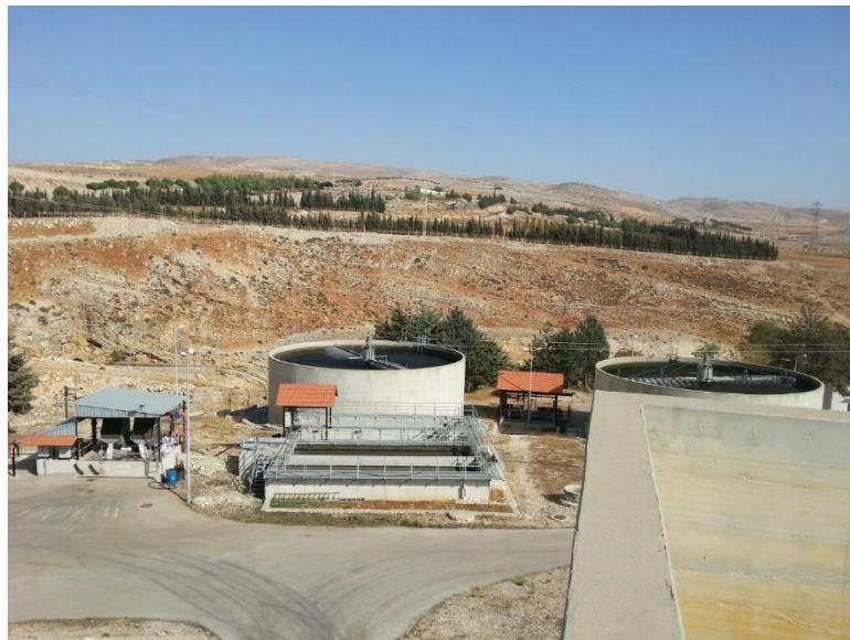
Figure 2-3 Two Trickling Filter Basins
